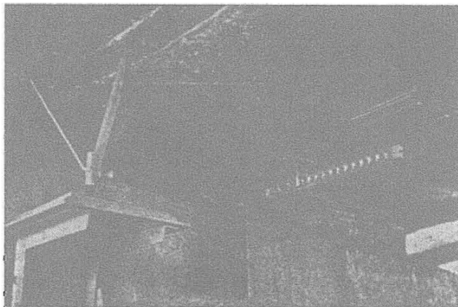
Figure 8 There can be value in arranging to place a device for measuring the width of a joint and the direction of the displacement. The above photo shows one possible solution (plans are available from the authors of this report)
